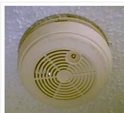
A residential smoke detector is the most familiar piece of nuclear technology for some people
