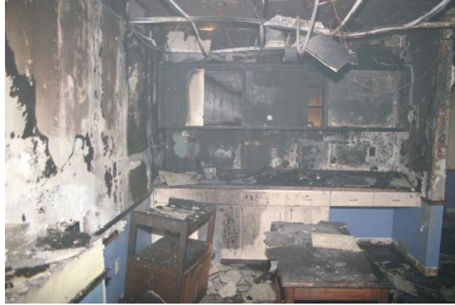
Figure 20.4 A fire in a kitchen. Note the V pattern of burning on the wall on the left side. Courtesy of James Novak.
