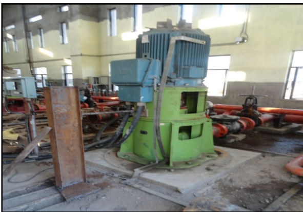
Fig. 1 : Measurement locations for vibration of fire hydrant pump.
