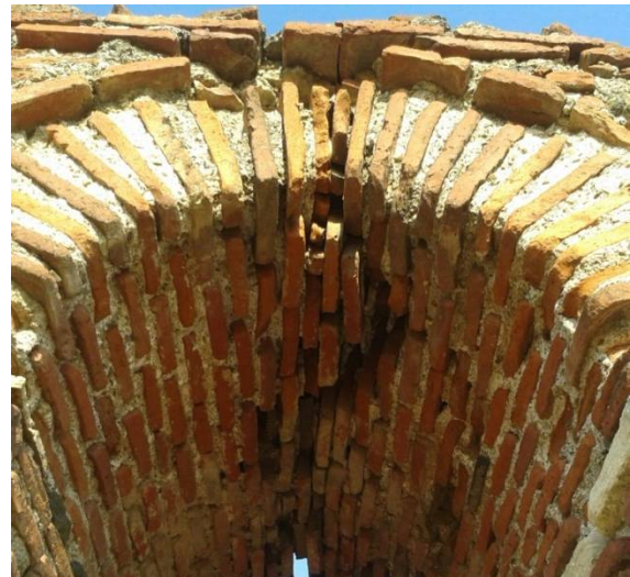
PHOTO 3: STRUCTURAL DAMAGES CAUSED BY SHIFTING FOUNDATIONS
