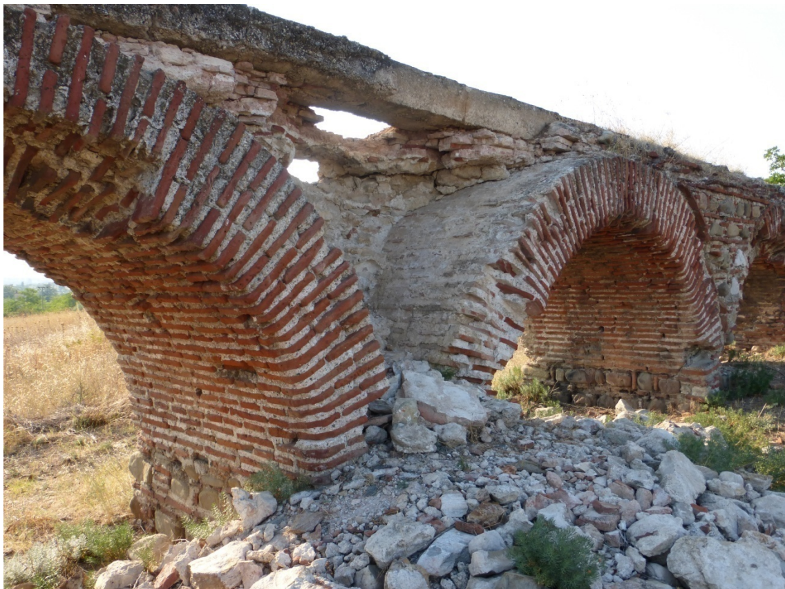
PHOTO9: DAMAGE TO THE BRICKS AT THE TOP OF THE AQUEDUCT AND BETWEEN ARCHES CAUSED BY FROST SHATTERING
