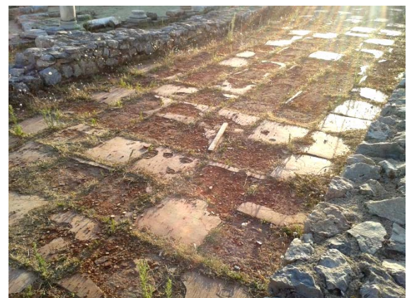
PHOTO 23: RECONSTRUCTED BRICK FLOOR ILLUSTRATES DAMAGE BY FROST AND VEGETATION
