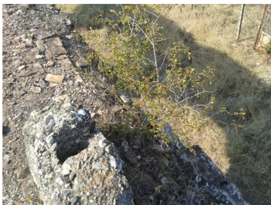
PHOTO 7: VEGETATION ON THE AQUEDUCT
