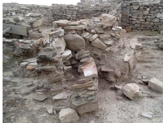
PHOTO 14: TIPPING OVER AND COLLAPSE OF EXPOSED WALLS FOLLOWING MORTAR AND PARTICLE EROSION
