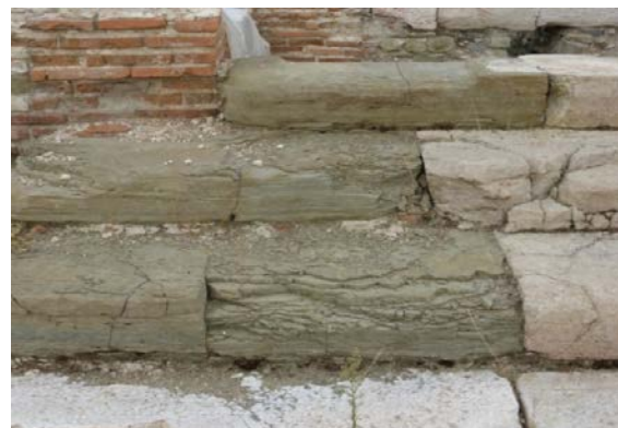
PHOTO 12: DECAY PHENOMENA ON DIFFERENT STONE MATERIALS
