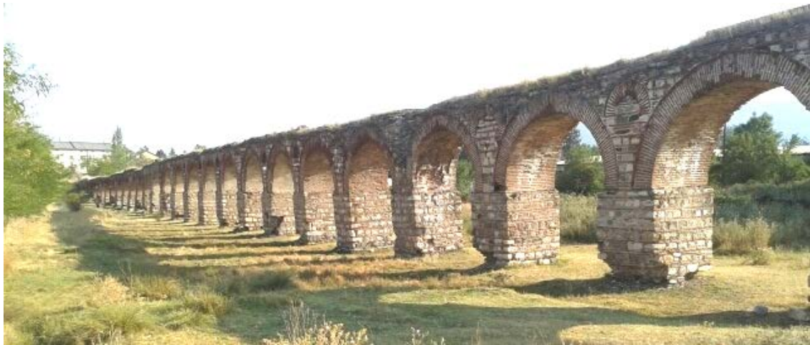
PHOTO 4: LEANING PIERS (CA. 19-27) IN THE SOUTHERN PART OF THE AQUEDUCT AFFECTED BY SOIL SETTLEMENTS
