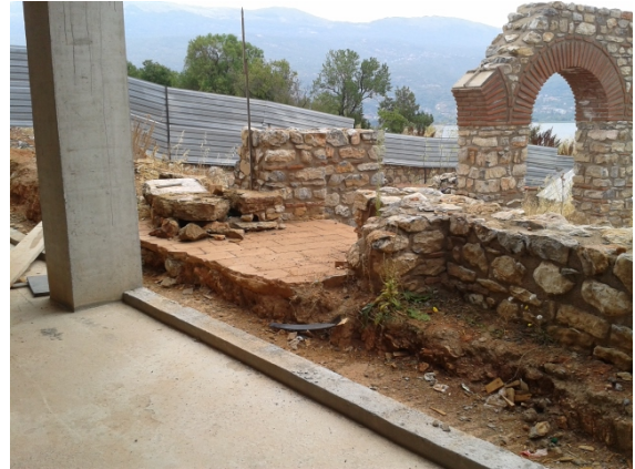
PHOTO 25: IMPACT OF NEW CONSTRUCTION ON ARCHAEOLOGICAL STRUCTURES
