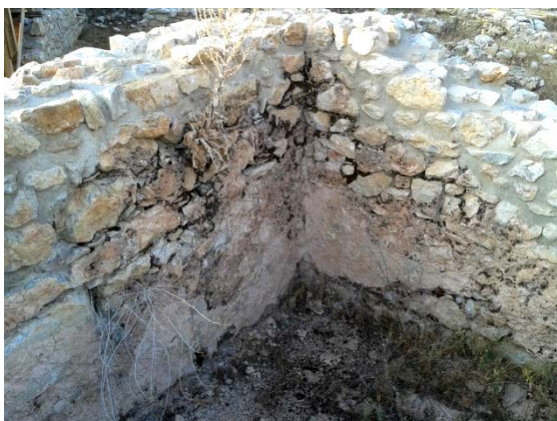
PHOTO 22: VEGETATION GROWTH IN HISTORIC WALLS UNDERNEATH LATER ADDITIONS
