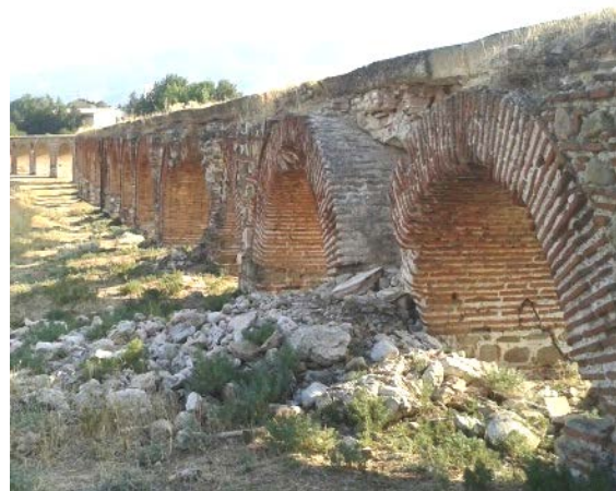
PHOTO 6: DAMAGES CAUSED BY FROST EXPANSION FOLLOWING RAIN WATER PENETRATION
