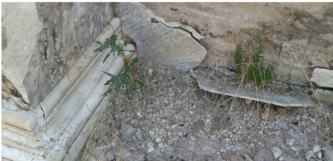
PHOTO 19: SEPARATION OF SURFACE LAYERS AS RESULT OF FROST AND VEGETATION
