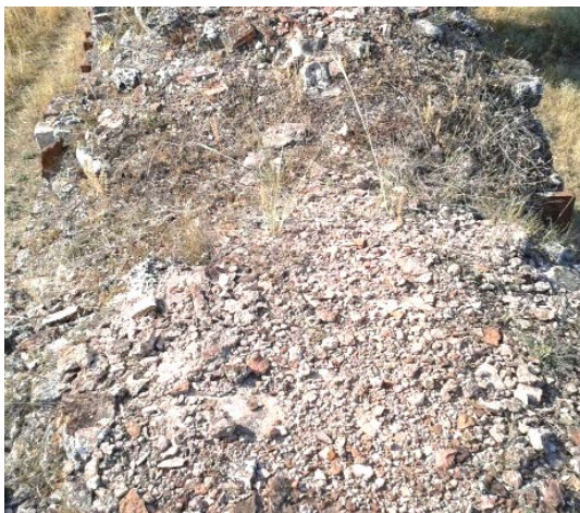
PHOTO 5: AQUEDUCT TOP SURFACE WITH DAMAGES CAUSED BY WIND AND WATER EROSION
