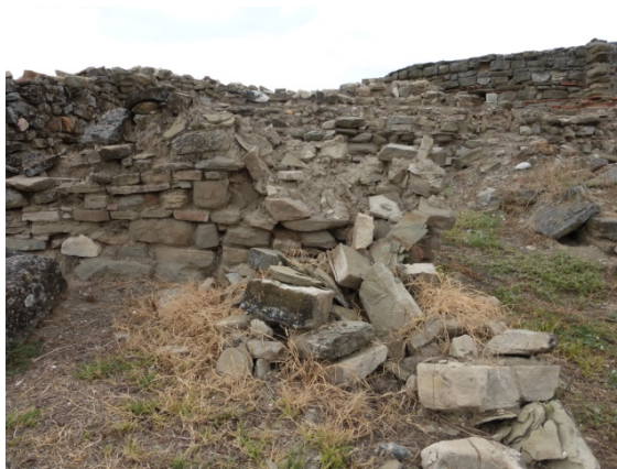
PHOTO 15: COLLAPSED WALLS CHANGING THE CHARACTER OF THE ARCHAEOLOGICAL SITE
