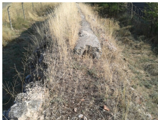
PHOTO 8: VEGETATION COVERAGE NEAR PIPE
