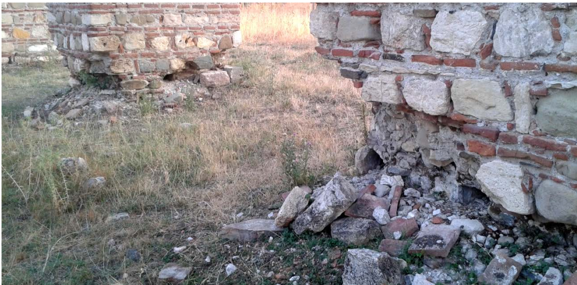
PHOTO 10: LOWE PIER AREAS WHICH ARE VULNERABLE TO FLASH FLOODS AND WATER EROSION
