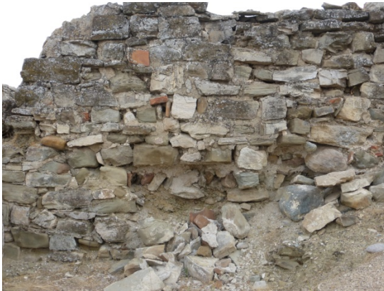
PHOTO 13: REMOVAL OF STONES AFTER BY THE LEACHING OF FINE-GRAINED PARTICLES
